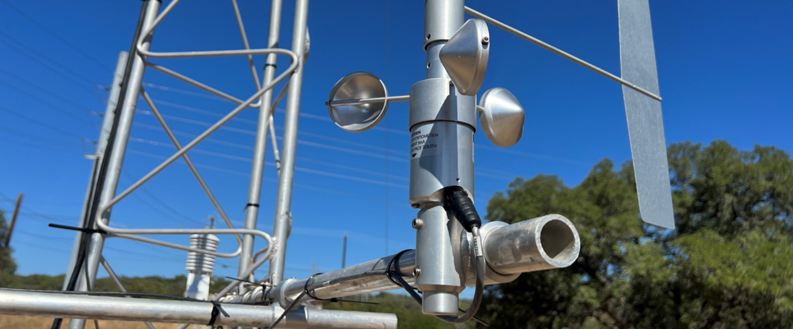
▲ The 100th TexMesonet station was installed at the Edwards Aquifer Authority's Field Research Park in northern Bexar County.
